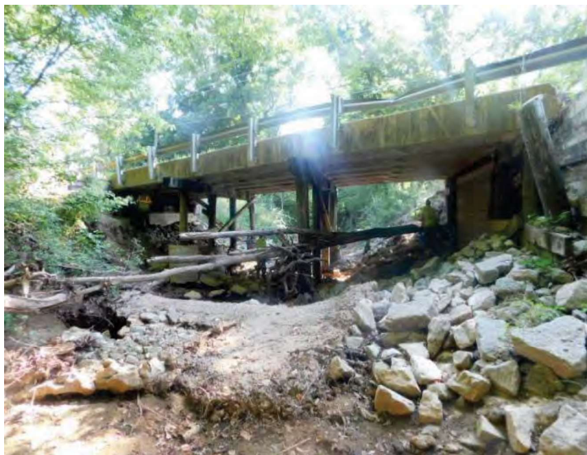
LEFT SIDE INLET END VIEW
