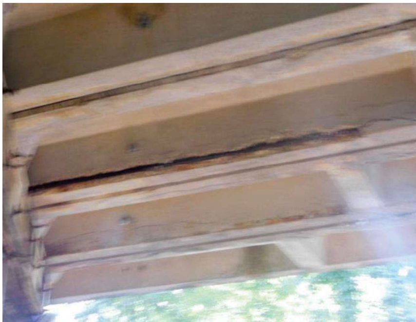
SLAB D SPAN 2 SPALLED TO STEEL
