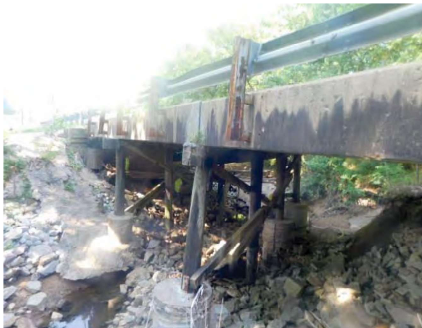
RIGHT SIDE OUTLET END VIEW
