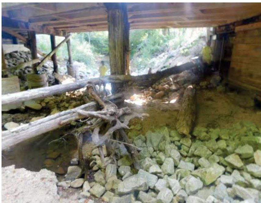
LEFT SIDE DRIFT INLET END
