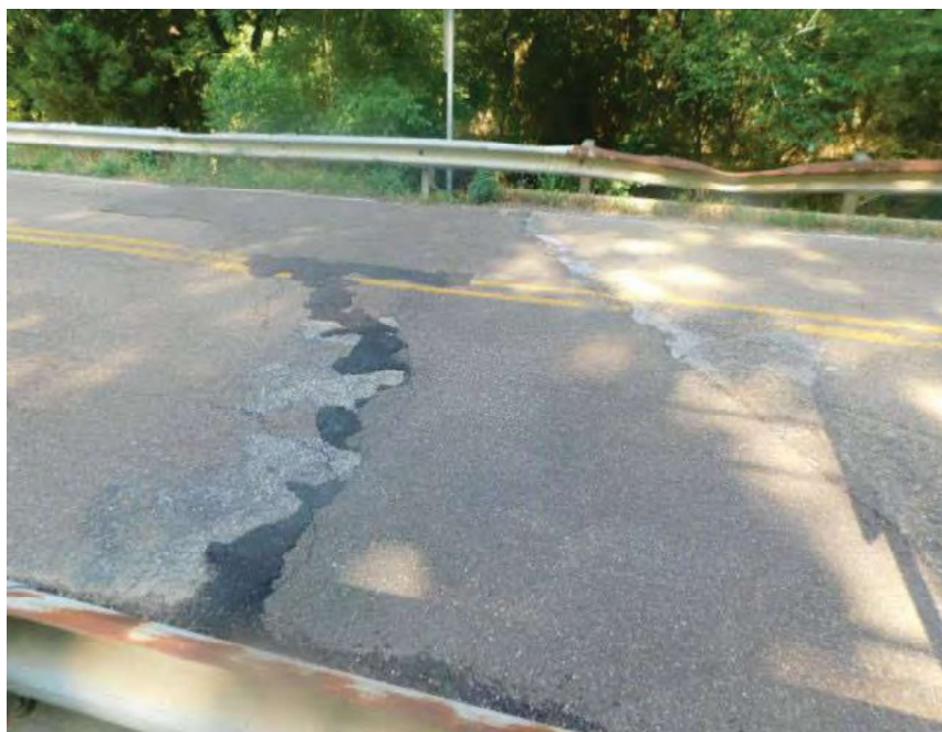
APPROACH 1 A/C PATCHED, CRACKED
