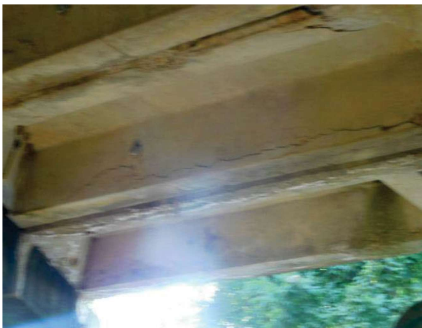
SLAB E SPAN 1 CRACKED
